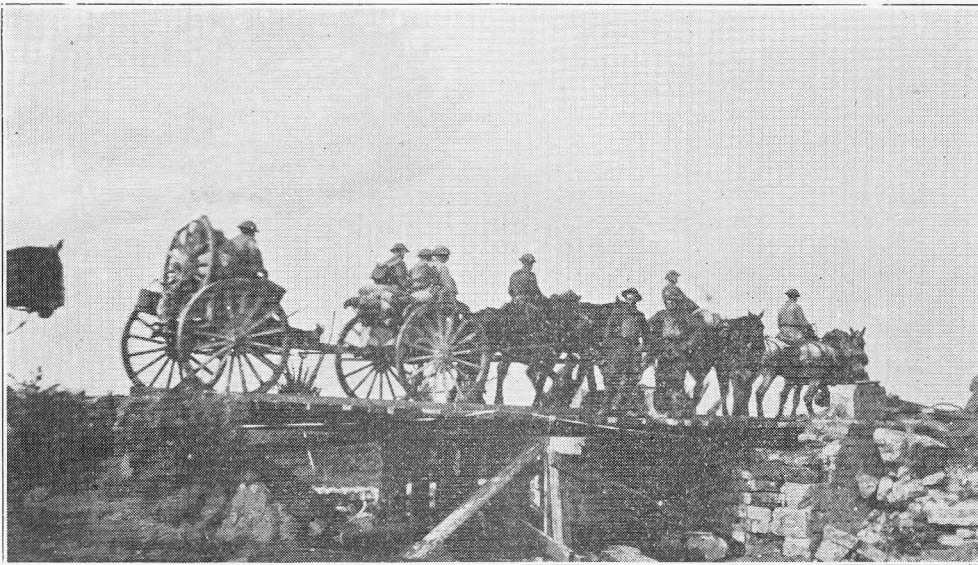
Bridge across Forges Brook at Bethincourt, constructed by Co. B., 305th Engineers, under shell fire on the morning of Sept. 26, 1918.
